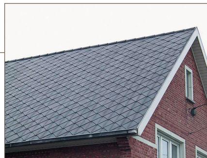
Dakleien in asbestcement
